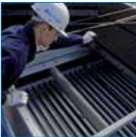
on site services
