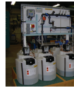
Water treatment equipment
